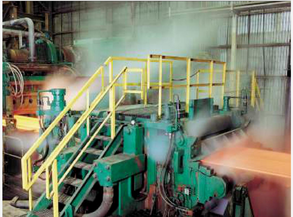
Descaler in front of a rolling mill of a thin slab casting mill
